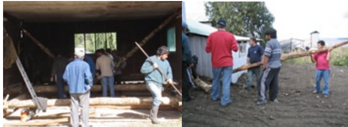
Reinforcement of the structure and Lifting off the house from its old foundations
